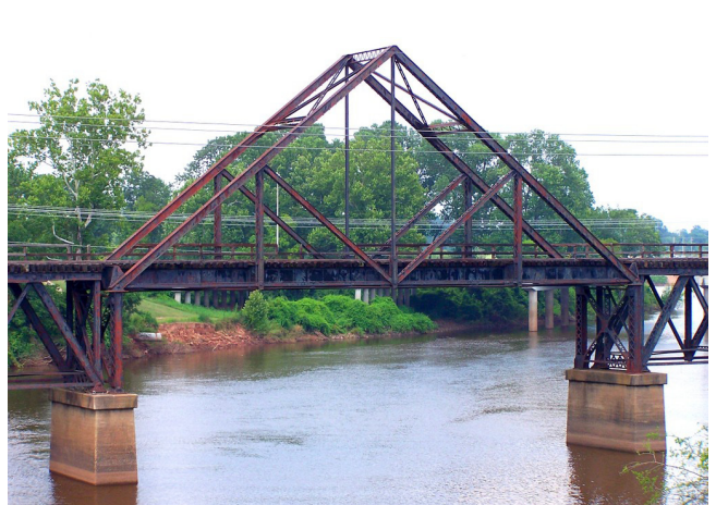
The distinctive silhouette of the Kansas City Southern Railroad Bridge over Cross Bayou, completed in 1926, marks it as a Waddell A-Truss railroad bridge. Only one other remains standing in the U.S.
